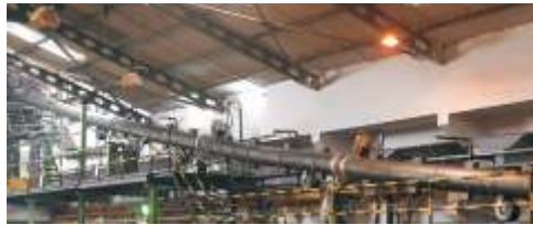
Figure 1: 6 Nos. CCV (DRY CURE) LINES
